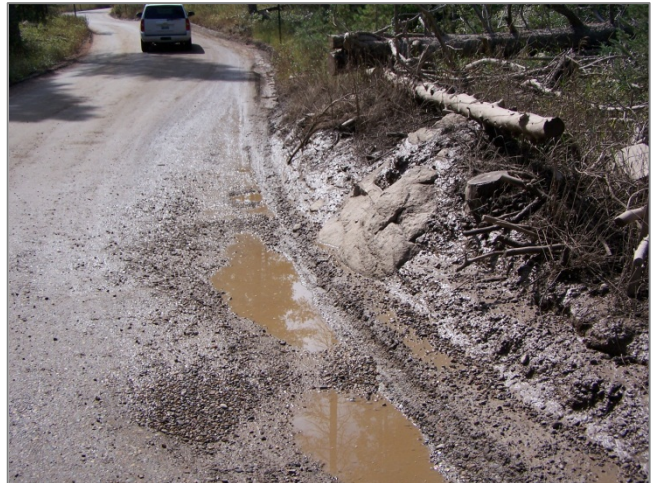
Figure 17. Unpaved Roadway and Roadside Hazards
